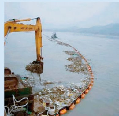
Trash boom installed in estuary area in Korea
